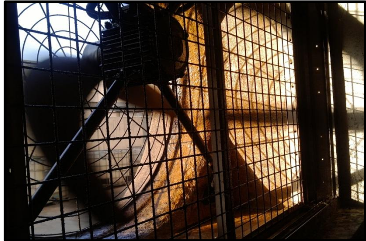
An oil-stained fan in the production facility
